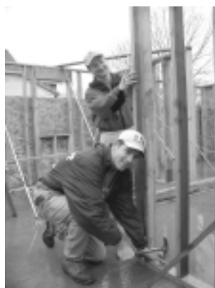
Watch that thumb! Rensselaer students work on the framing for a house.
